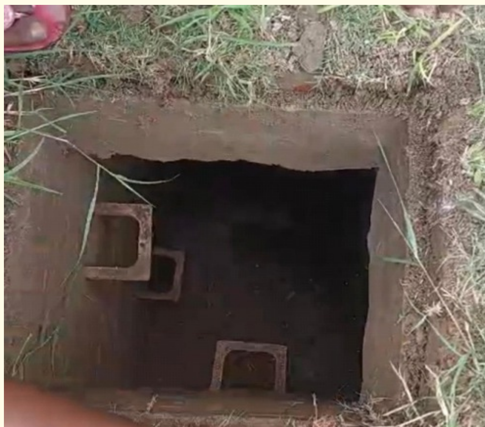
Rainwater harvesting pit at FDDI, Rohtak Campus
